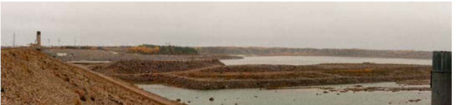
Photo 41: Limestone Hydro-electric Generating Station and its cofferdam, September 2016. (Photo Credit: Victoria Grima)
