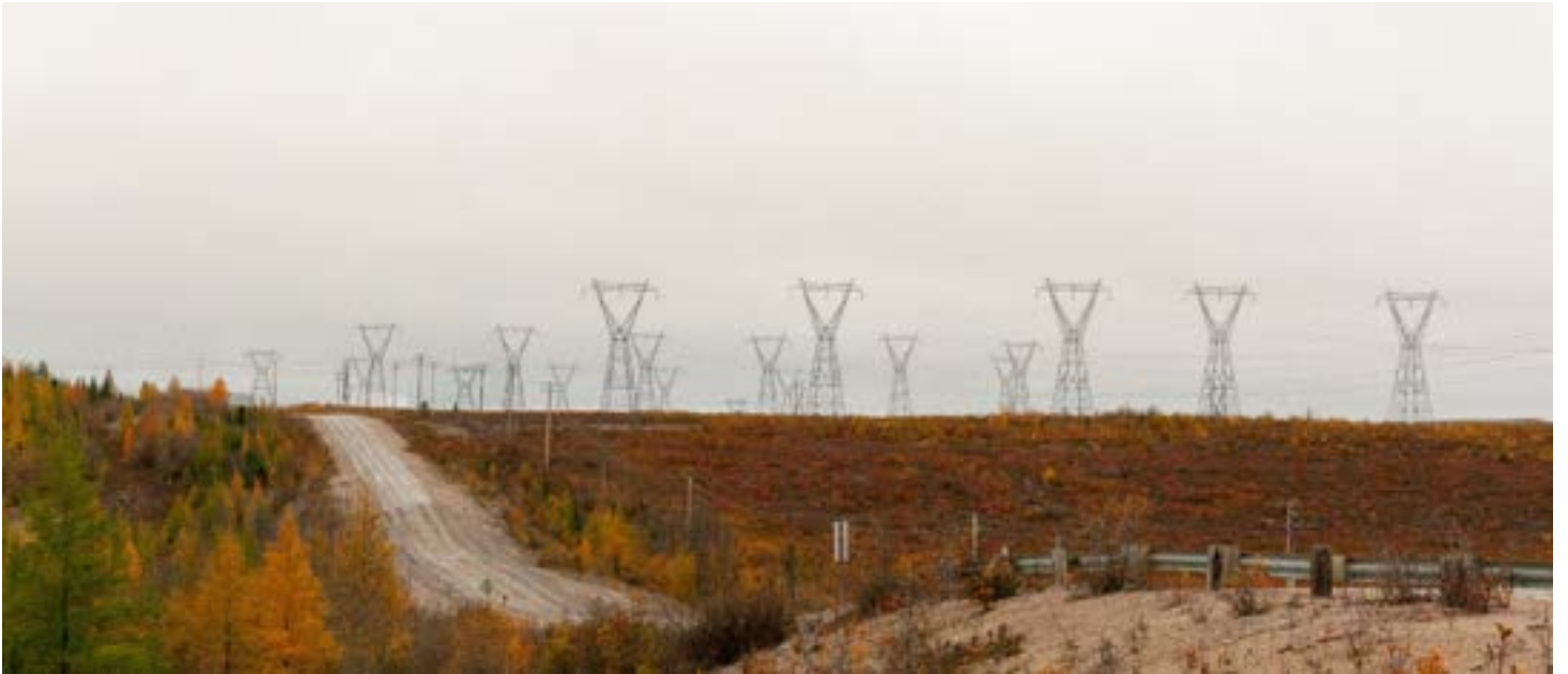
Photo 33: The high-voltage towers carrying the generated hydroelectricity by Long Spruce GS, September 2016. (Photo Credit: Victoria Grima)
