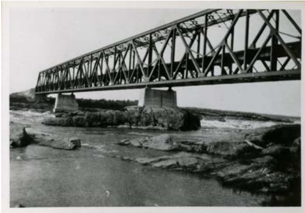
Photo 23: undated view of Railway Bridge over Kettle Rapids. (Retrieved from University of Manitoba, Libraries Online Digital Collection, Nan Shipley Fonds, Northern Manitoba Album 1, URL https://digitalcollections.lib.umanitoba.ca/islandora/object/uofm%3A11493/manitoba_metadata )
