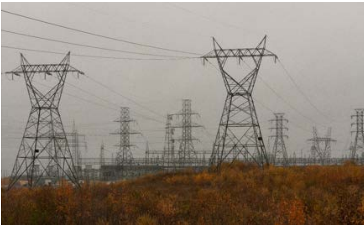
Photo 38: Henday CS surrounded by the high-voltage towers, September 2016. (Photo Credit: Victoria Grima)
